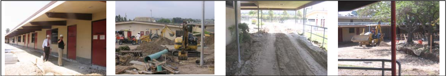
Bob Collins, Superintendent and Steve Coover, Principal tour the construction at Mount Miguel High School
